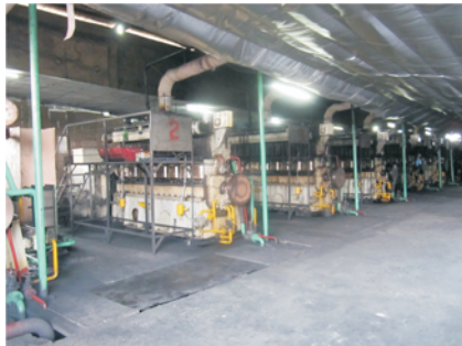
Biomass power plant using rice husk
