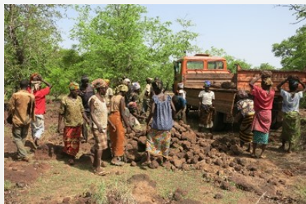
One of 60 working groups loading stones for various construction purposes, such as stone rows and dikes. The average protected soil surface due to erosion measures is about 5,000 ha per year.
